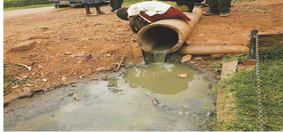
Figure 4: Burst sewage tank in Budiriro suburb of Harare City, 2011
